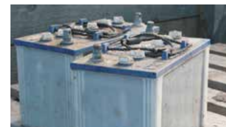
Fig. 46: Examples of bad used lead batteries management
