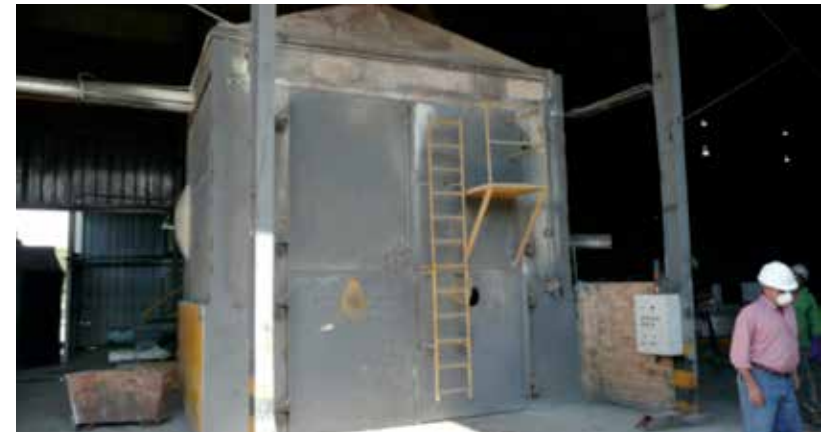
Fig. 27: Furnace of Industrias Meteoro S.A. - Dominican Republic 25 .
